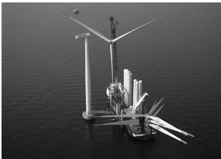
Figure 2.5: Erection of a wind turbine at the Nysted offshore Wind Farm (72 x 2.3 MW Bonus) commissioned in 2003
